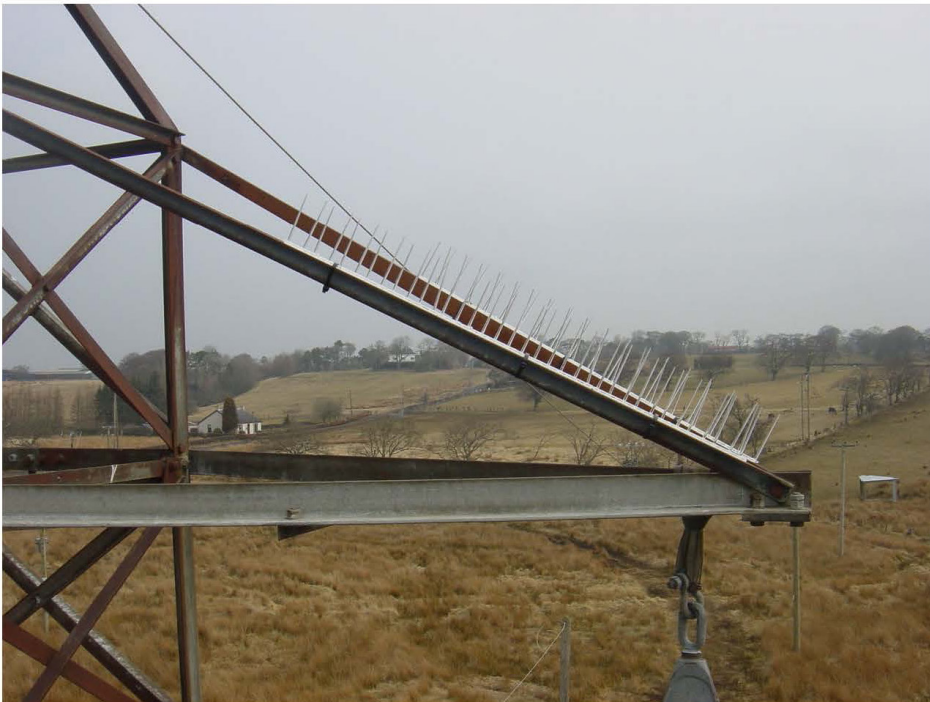
Fig 7 Bird Deflectors Fitted to a Tower near the Landfill Site
