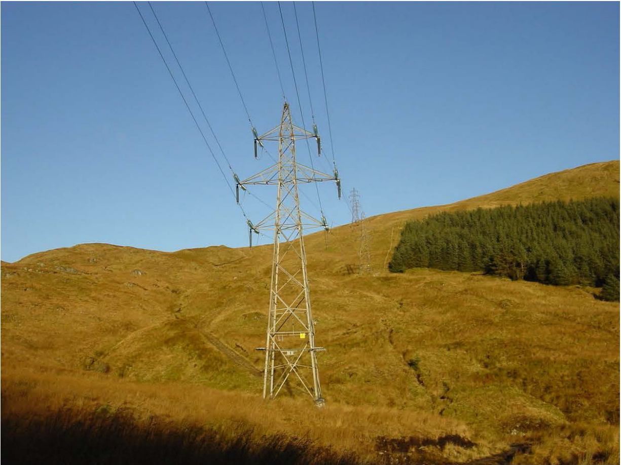
Fig 2 132KV Tower on the Dunoon Tee
